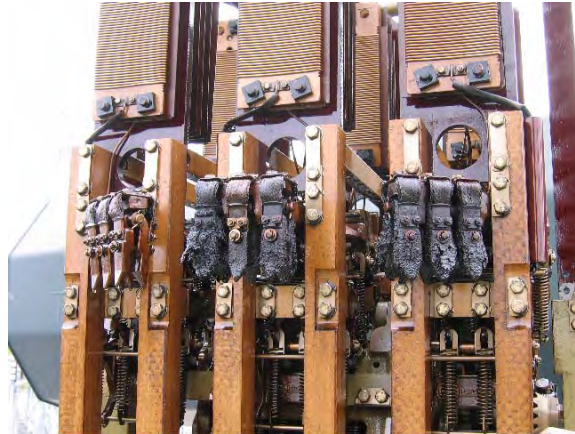
Figure 1: Example of heavy coking on LTC contacts 28
